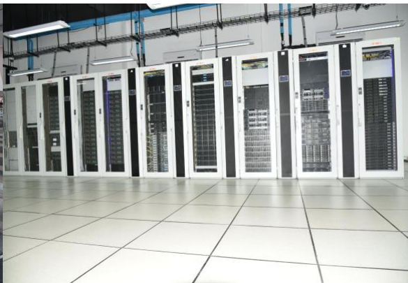
ICTS Data Centre
