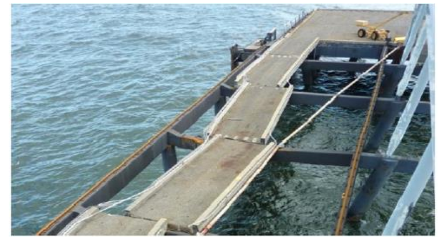
Damage to Lucinda port during cyclone Yasi, 2011 (Burston et al., 2012)
